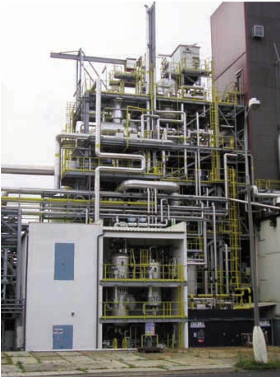
The new entrained flow gasifier installed at the Vresova IGCC facility. It gasifies plant by-products to generate syngas. This is fed to the two combined cycle units. (Photograph courtesy of Sokolovská uhelná)
