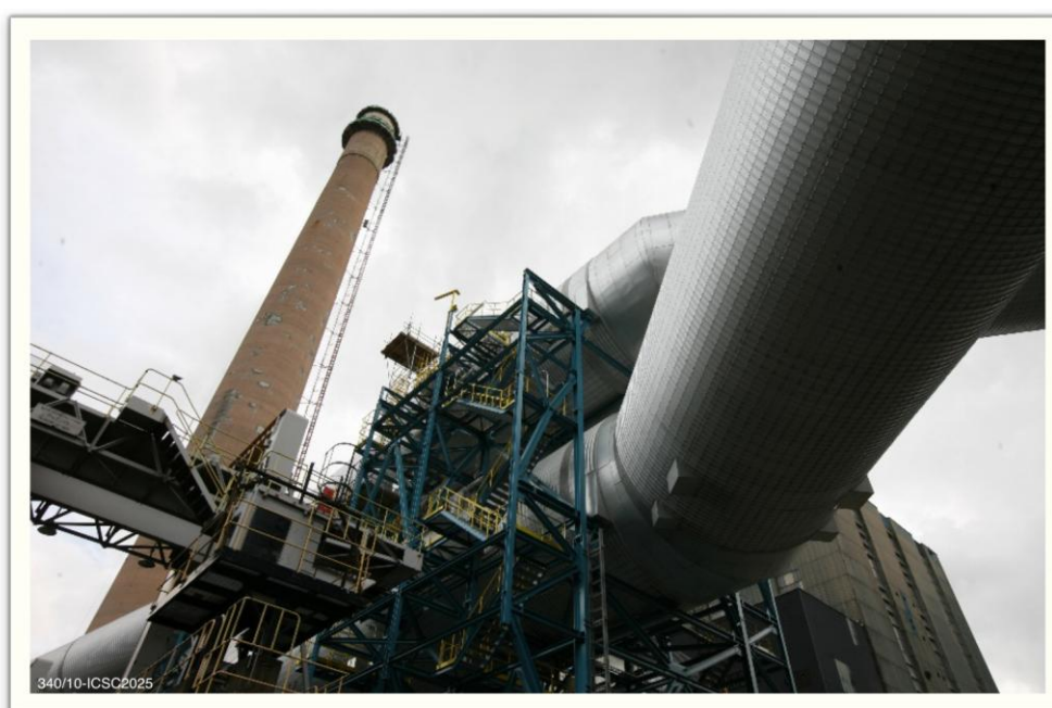
Figure 10 FGD unit on UK coal-fired power plant (courtesy of Russell Mills Photography)
