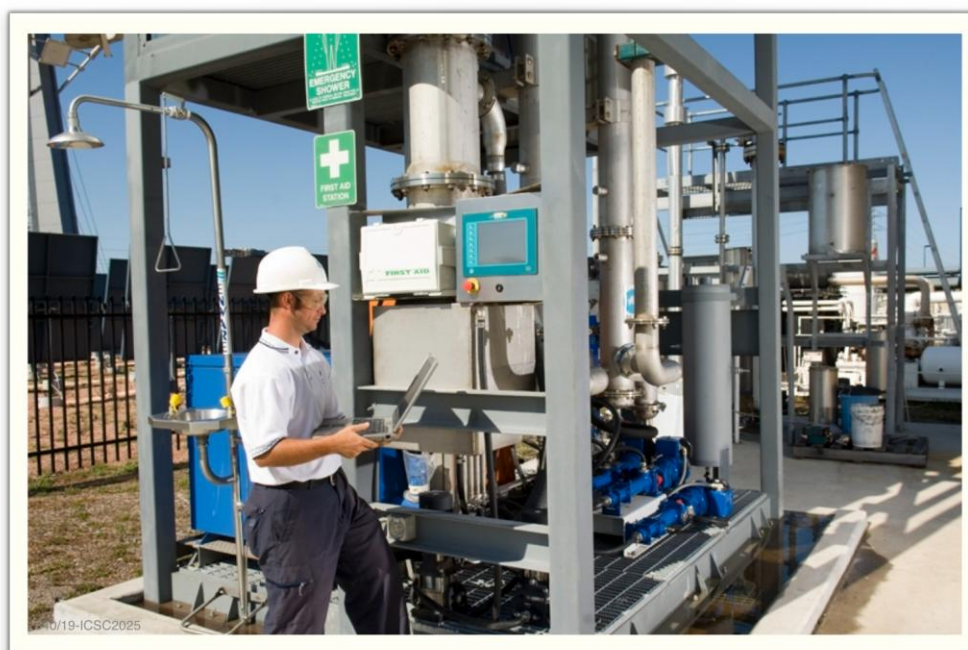
Figure 19 CSIRO amine-based post-combustion pilot project, Loy Yang, Australia (courtesy of CSIRO)
