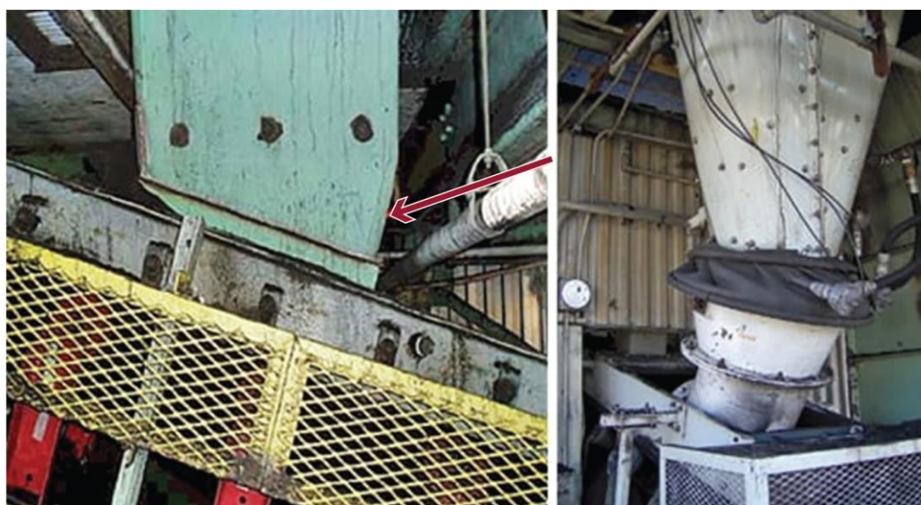
Figure 9 Fuel-handling equipment upgrade at Big Brown power plant, USA – InteliFlo® system (Image courtesy of: Power)
