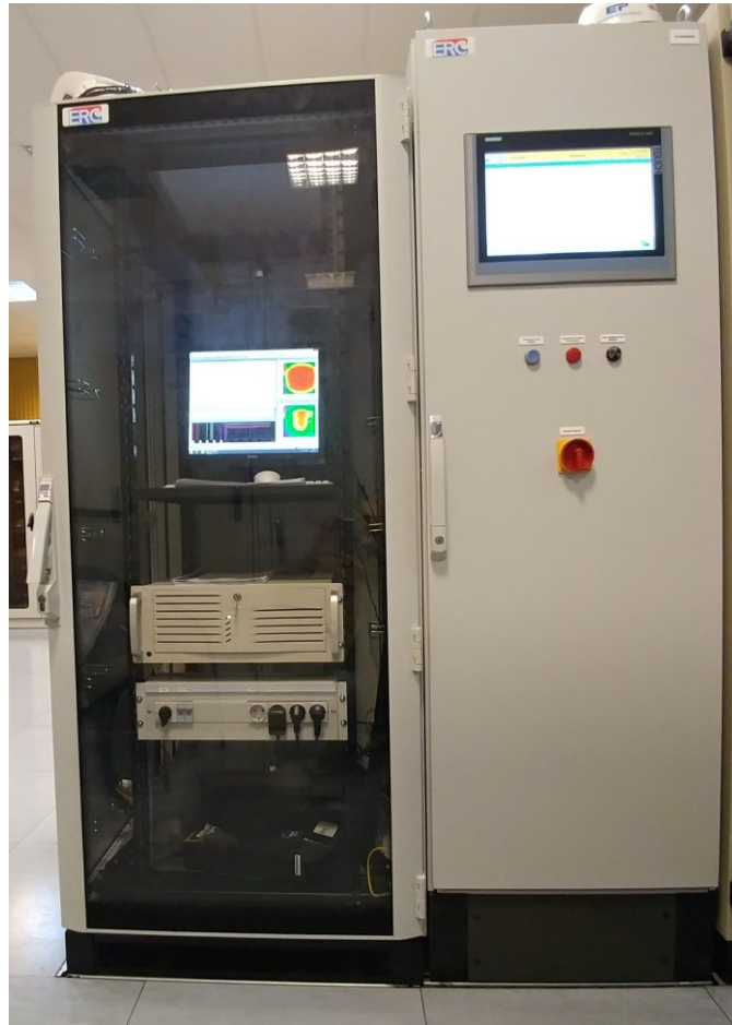
Control Cabinets of SNCR and for Temperature Mapping System
