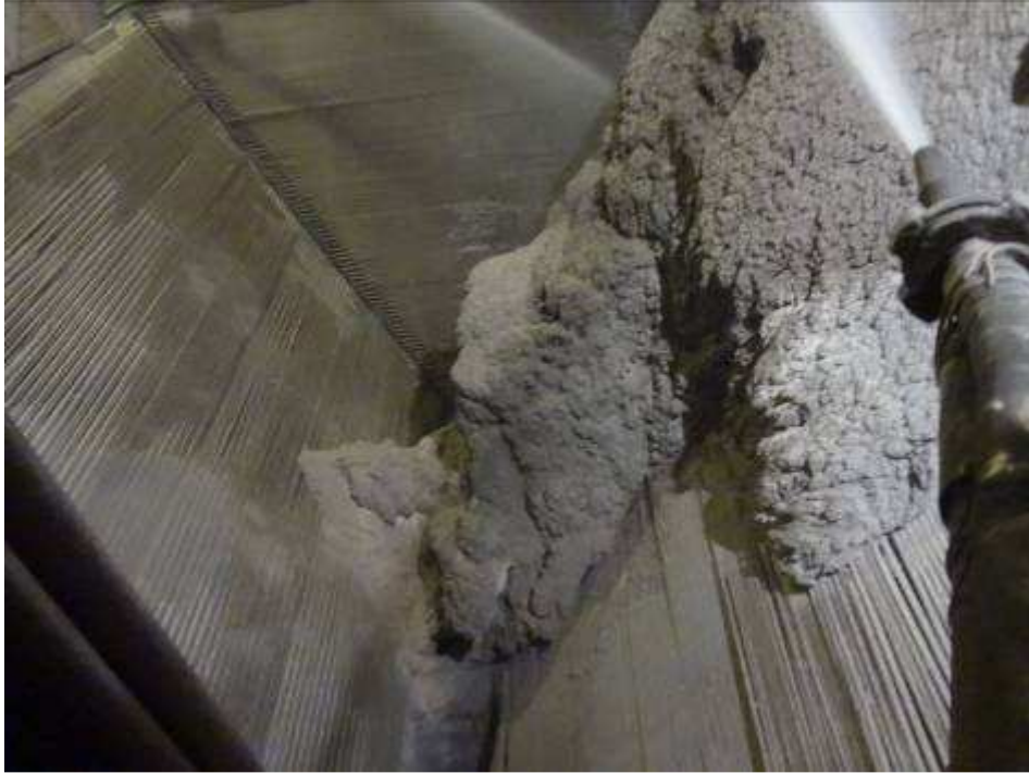
Figure 2 – Furnace hopper plugged by slag accumulation
