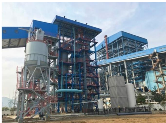
China's first biomass cofiring pilot project at Xiangyang coal-fired power station (Courtesy of China Hefei Debo Bioenergy Ltd)
